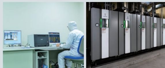
Central control room
