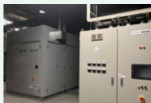
A refrigerator that uses natural refrigerant (Mie Plant)
