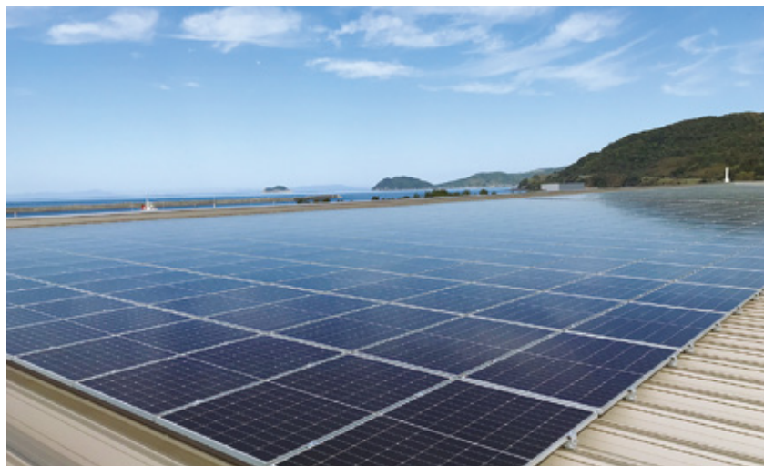
The plant's solar panels cut its annual emissions by more than 5,000 tons.
