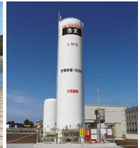
For boiler fuel, the plant uses LNG, which has a low carbon footprint.
